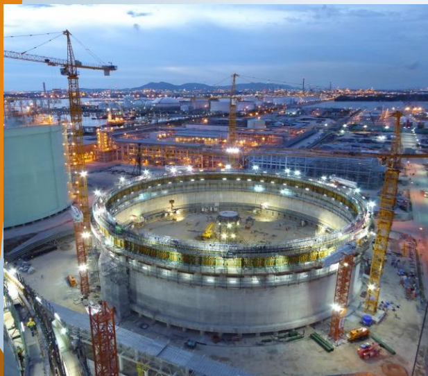
▲ Aerial view of the two LNG tanks
